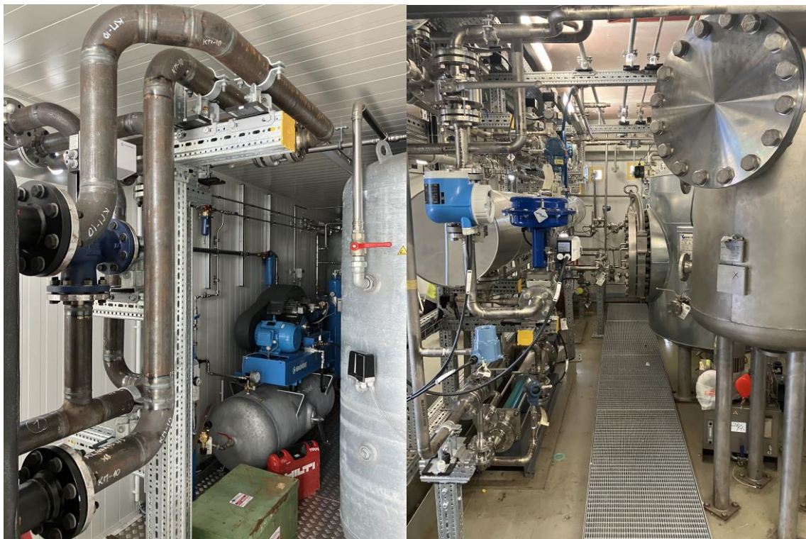
Figure 4. Utilities nitrogen and cooling water
